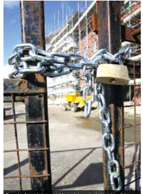
Breach of regulations could result in a site being closed down.
